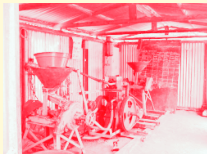
The basic energy infrastructure of the Platform consists of an 8 hp or 10 hp (approx 7 kW) diesel engine (the Indian-made Lister engine, widely available in rural areas of Mali and Burkina Faso). (Photo: Multifunctional Platform, Mali)
