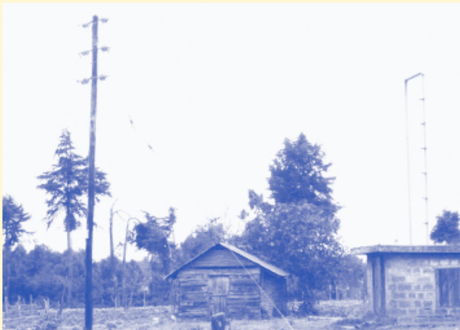
Medium voltage power cables used in Njambine, a rural town in central Kenya (Photo: AFREPREN)
