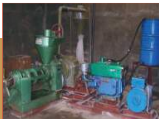
The multifunctional platform installed at the Nyantonzi project site.
