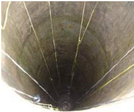
Photo 1: A water well
