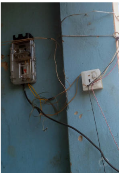
Wiring before upgradation
